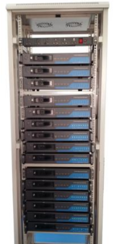
Multiple devices in the rack
